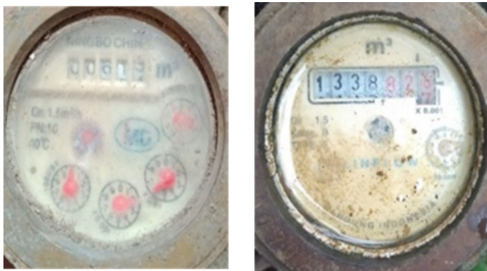
Figure 12: Examples of water meter that reads incorrectly.
