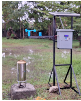
Figure 5: Rainfall sensor and landslide EWS.
